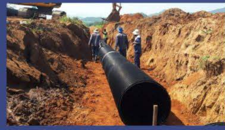
Wastewater/Sanitary sewer Pipes
